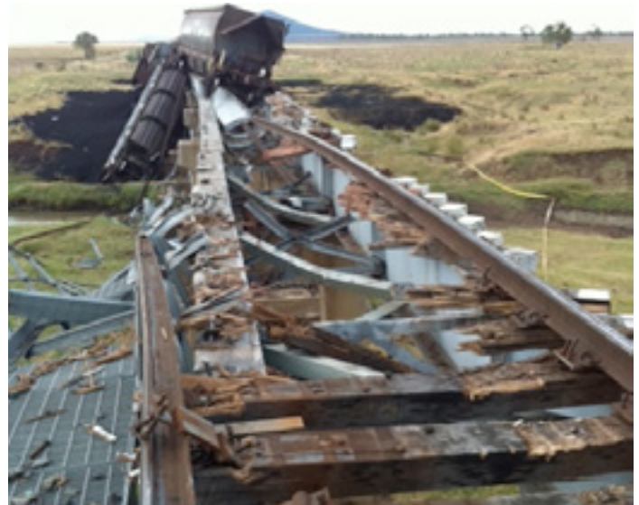
Boggabri Coal Train Derailment - Rail line out of action.
